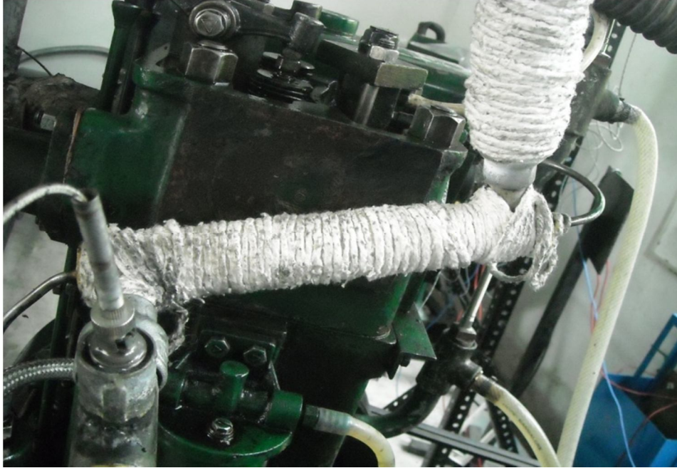
Figure 3.10: Heat Exchanger installed on the engine fuel supply system
