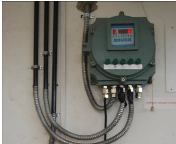
Figure AE.13 Hydrogen gas monitoring system
