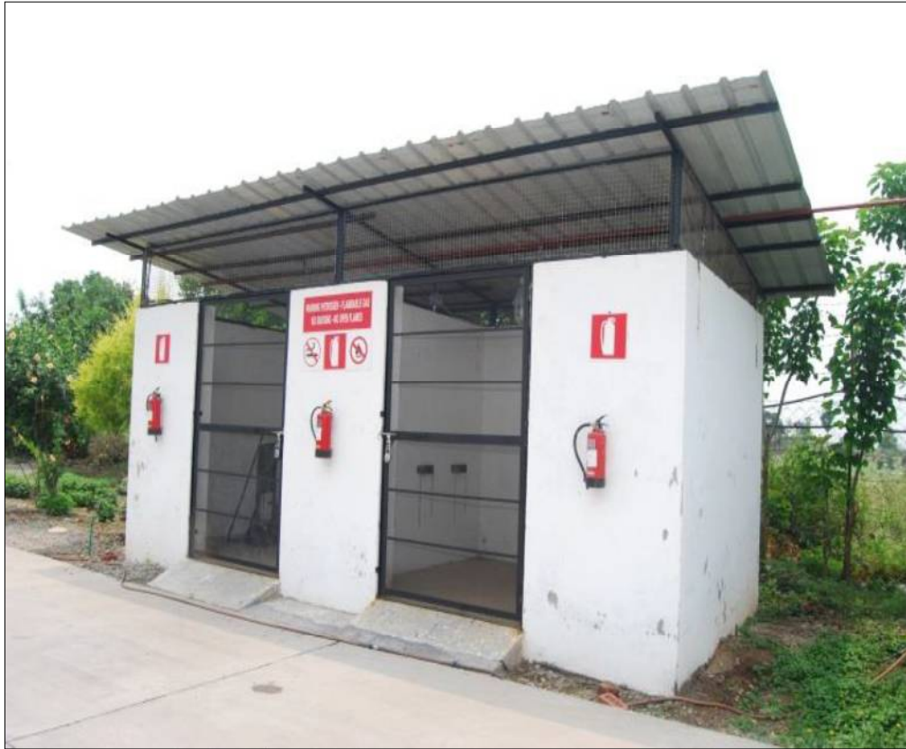
Figure AE.15 Hydrogen storage area
