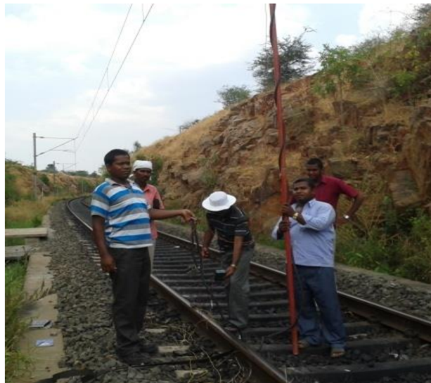
Fig.4.5 Data collection from the actual high voltage traction line at railway earth cutting
