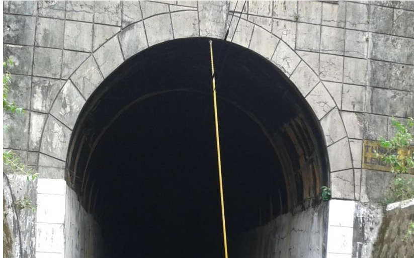
Fig. 6.4 Bare conductors of OHE run close to earth potential surface
