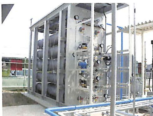
Gas Storage Unit
